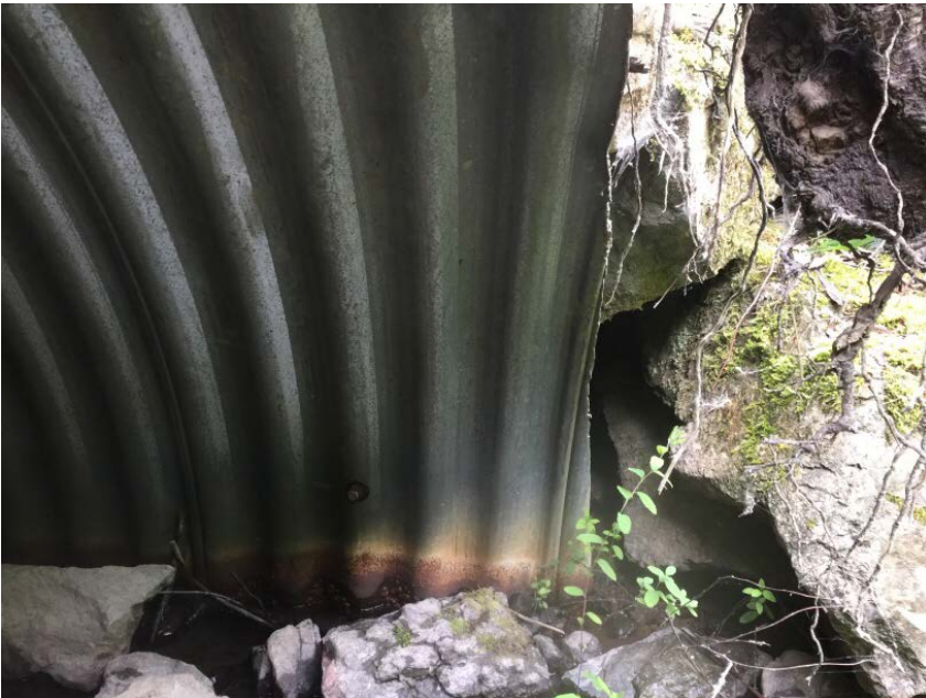
Minor corrosion on culvert noted
